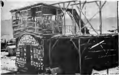
Figure 55. Structures can be made to conform to the architecture common to the locale by erecting super-structures of light timber and covering them with burlap, plaster, or other material. Here, a quonset hut is being altered to resemble the surrounding native houses.
